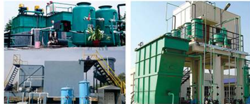
EFFLUENT TREATMENT PLANTS
